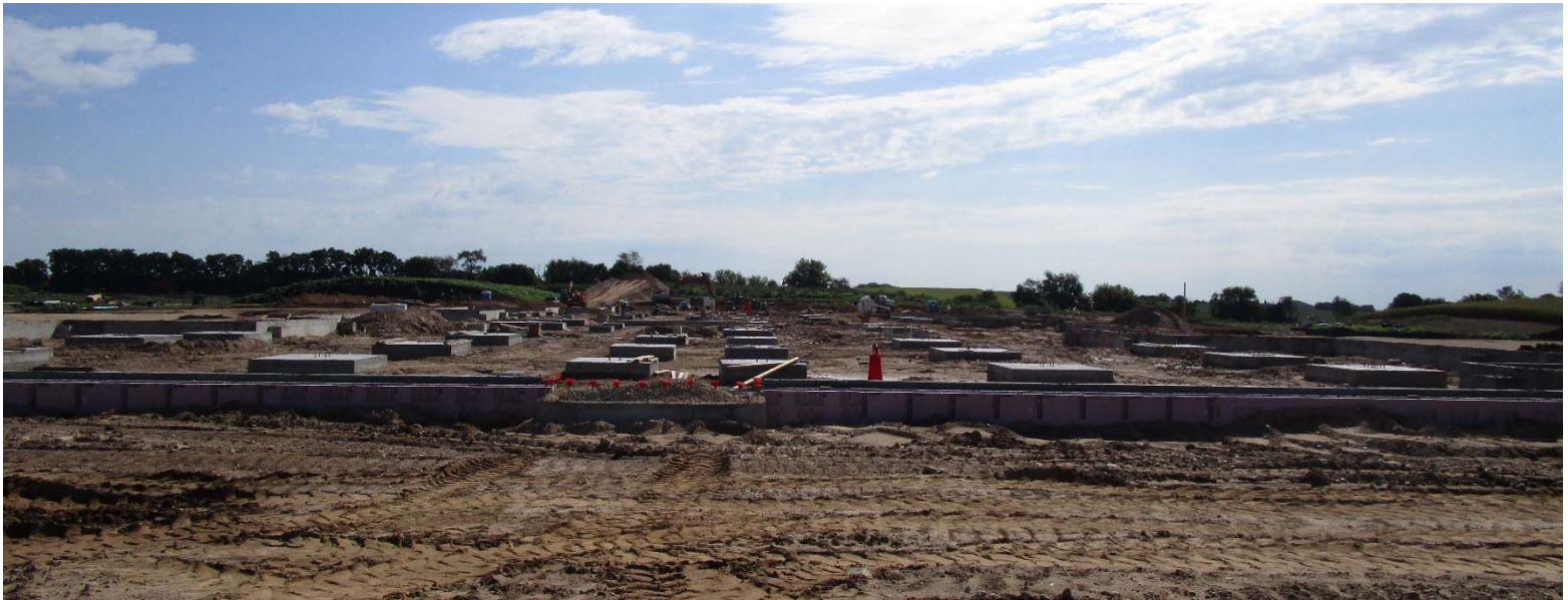
All of the concrete pads from the view of Area A. The foundation and exterior wall insulation is also pictured for section A.
