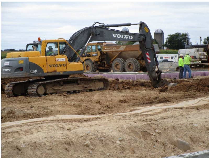
This large piece of equipment is an excavator, and is doing the backfill on the south side of the school.
