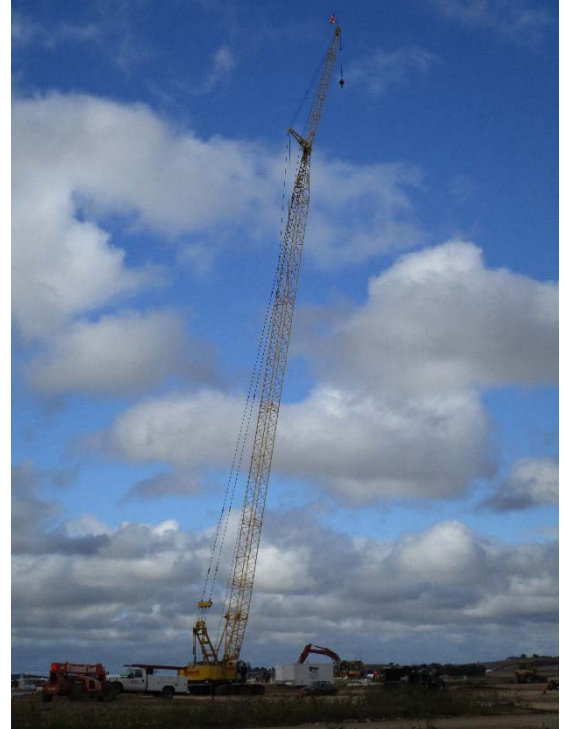
The Findorff crane has been brought to site to begin structural steel erection on Monday. The 100 ton crane is currently 250 feet tall!
