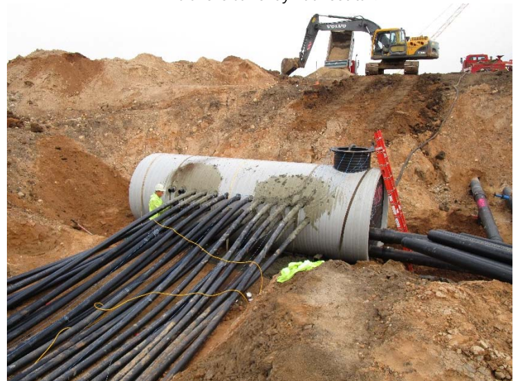
Most of the pipes are attached to the vault, and on the left is the supply and return line to the school building.
