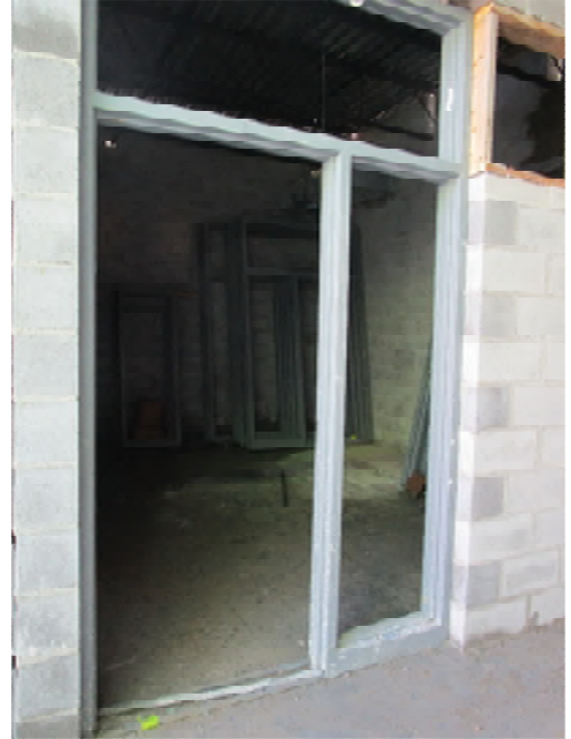
Some hollow metal frames were delivered last week and a couple have been installed in rooms with masonry walls.
