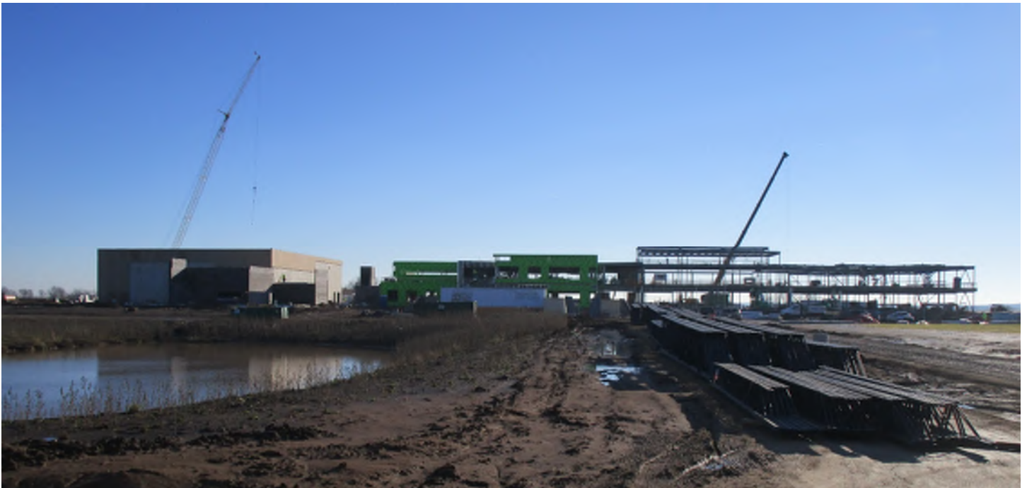
Progress of the overall school with many studs in B completed and covered with sheathing. Check out real-time video on Waunakee Community School District's website under building progress.
