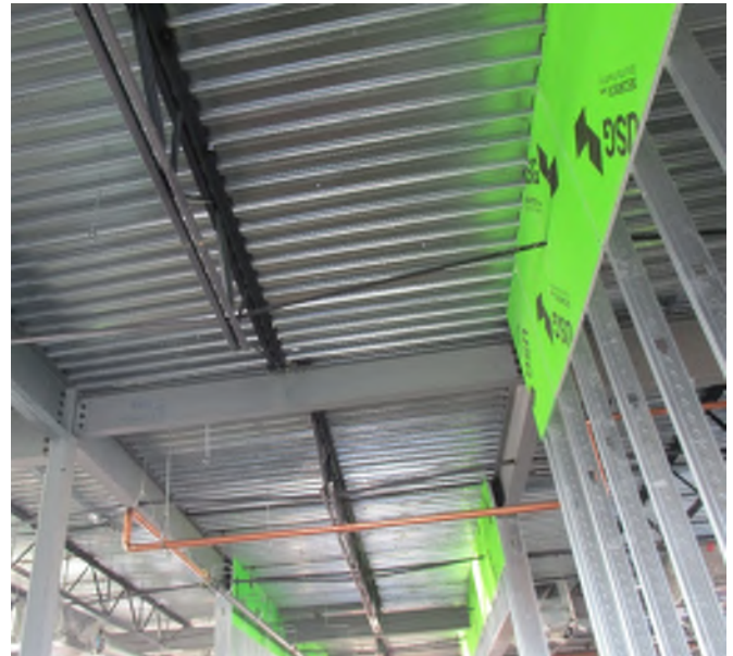
Much of the steel decking is done in B, providing some protection for the winter weather experienced onsite!
