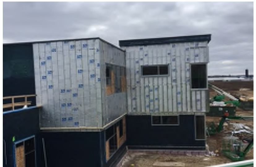
The framing you see in this picture are called furring strips and will be used to support the metal panel building skin.
