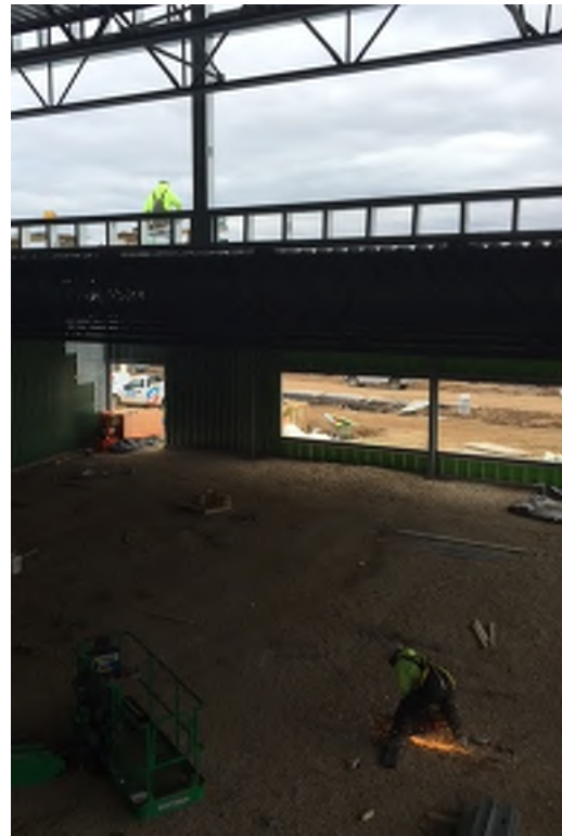
A dual action shot with ironworkers finalizing steel in The cafeteria and roof blocking overhead on the roof.
