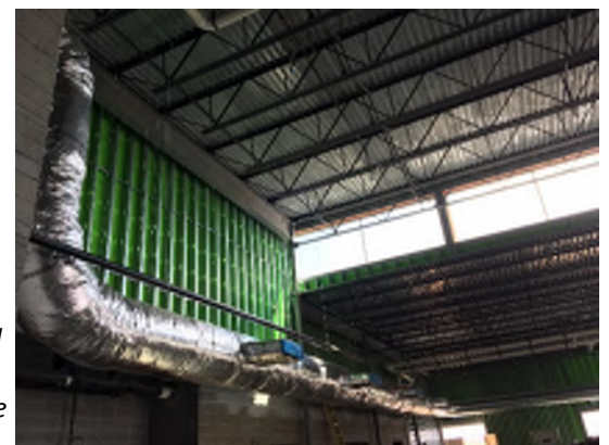
Giant HVAC duct set in the cafeteria area
