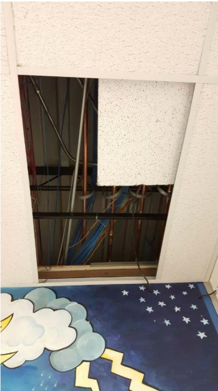
Globalcom has moved a ceiling tile so that they are able to get a head start on running their cable.
