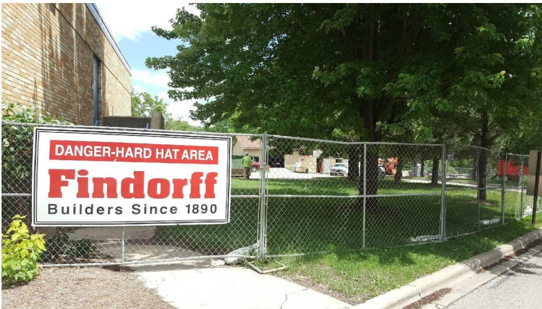
Findorff has set up a hard hat area in order to protect all of the people at Heritage Elementary.
