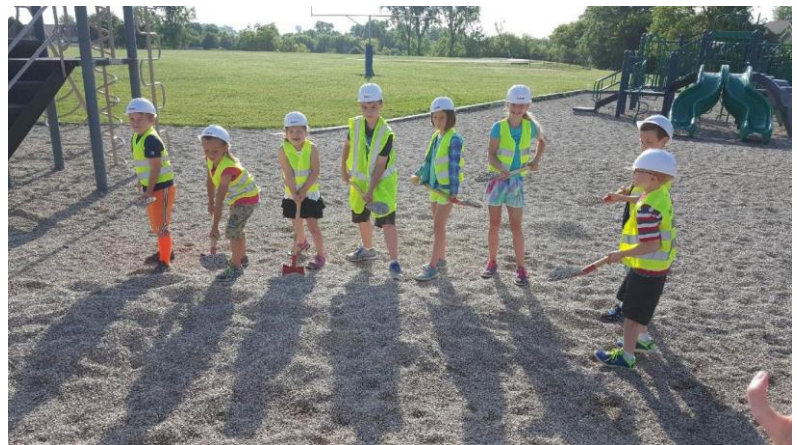
Eight happy students help Findorff break ground by removing the Pea Gravel from the existing playground.
