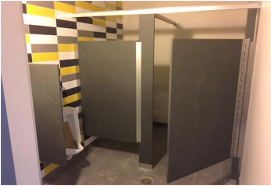
With the installation of toilet partitions, the bathrooms on the second floor are nearly complete (above).
