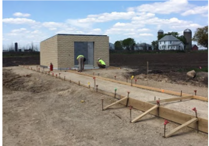
The equipment shed is built and the sidewalk near the lacrosse field is ready for concrete.
