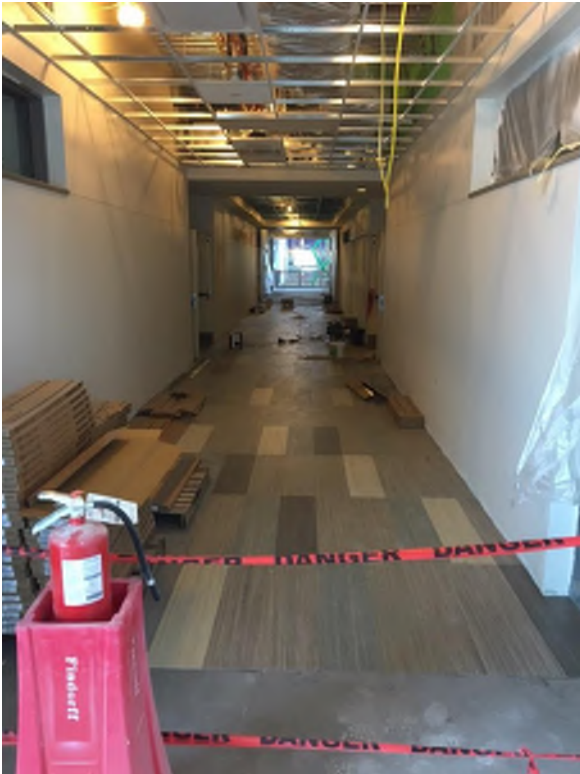
Area 2B is currently blocked off to everyone to allow the resilient flooring tile to set (below).
