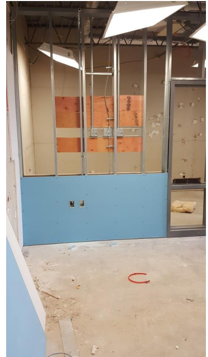
Drywall is starting to be hung in room B105. You may notice that there is also plywood hung on the wall. This is for the TV's that will be installed!
