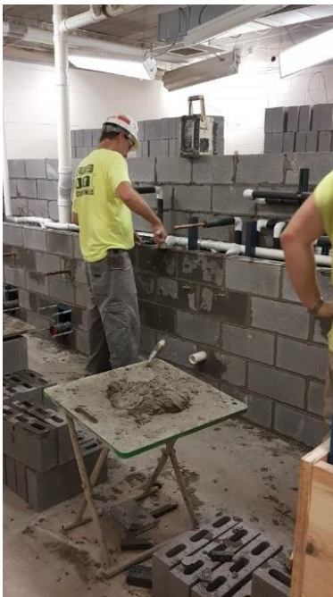
Masons are hard at work laying the bricks for the wet wall in the remodeled bathroom.
