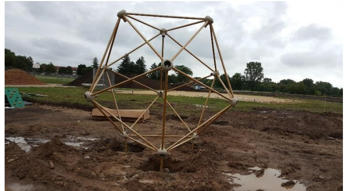
This is just one of the many new pieces of playground equipment that is being installed. They all look so fun!
