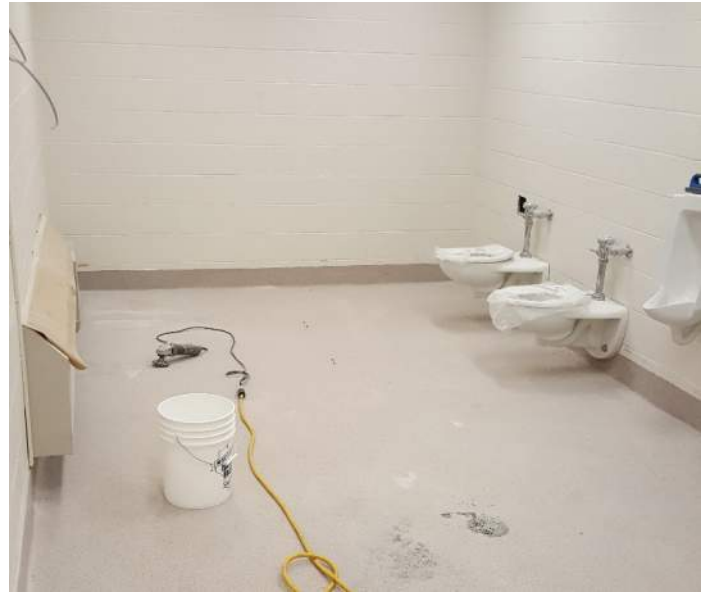
Epoxy Flooring was set in lower level bathrooms B009 & B013 this week.
