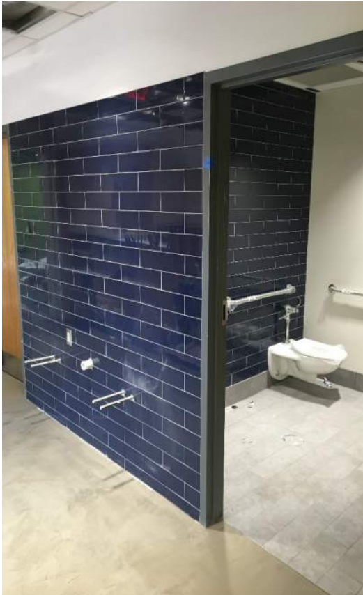
This "Sapphire Bright" ceramic tile color really looks sharp! This is toilet room C011C next to the shared resource area.
