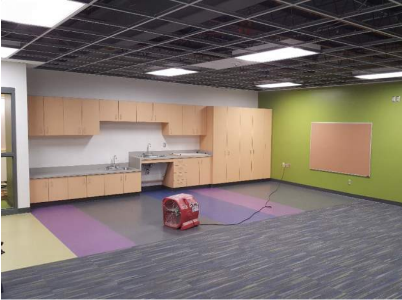
Lots of finishes went in this week in classroom C021. This includes casework installation, epoxy flooring, final painting and carpet.
