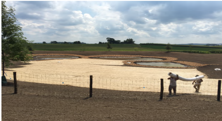
The Bruce Company finishing up the storm water pond at the back of the site
