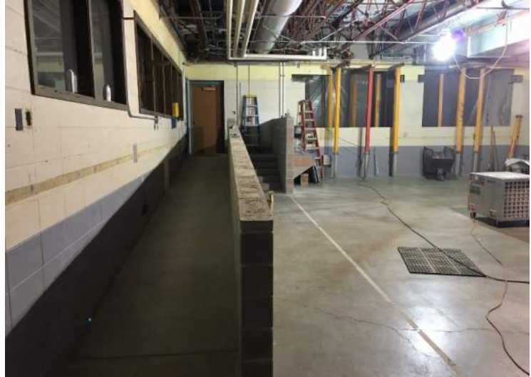
New masonry walls, ADA access ramp poured, stairs, sink, and windows cut out and shored at the corridor!
