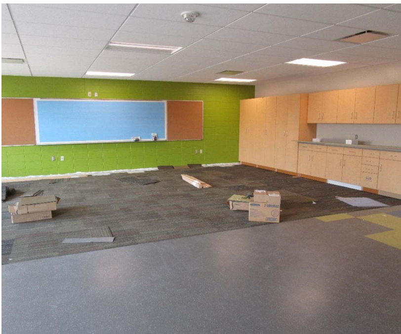
Visual display board on the accent wall, with new tile carpet and resilient flooring just installed in the new kindergarten classrooms.
