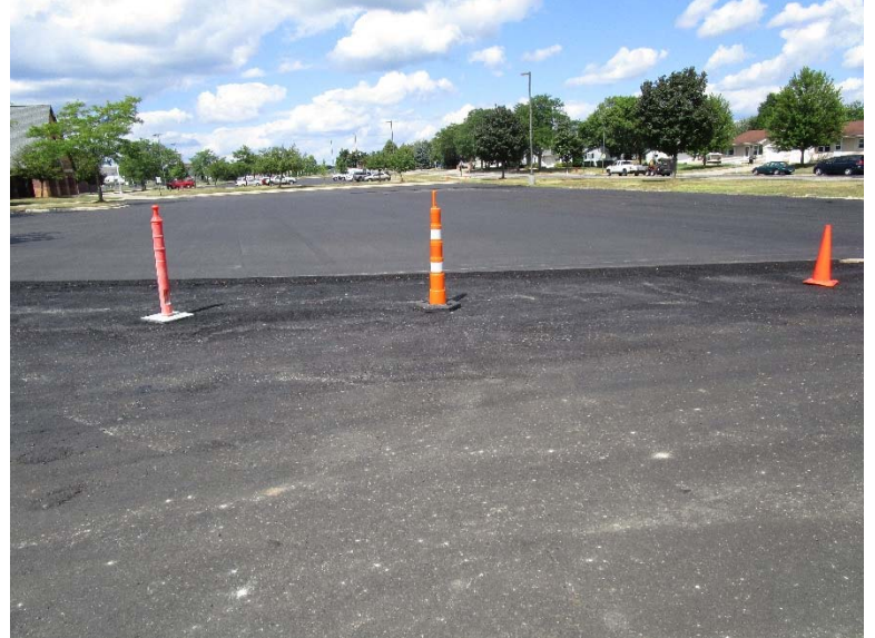
Parking lots in front of the building were also completed. Final course of asphalt and striping after completion of playground equipment.
