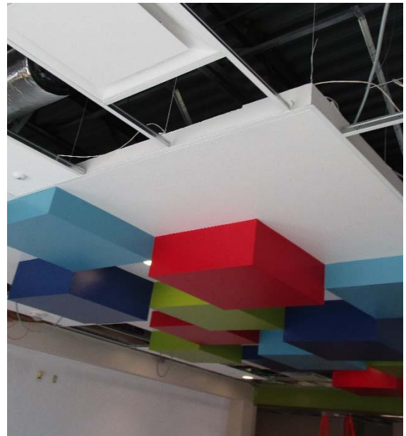
Ceiling detail in the new breakout area with paint colors to match the classroom accent walls.
