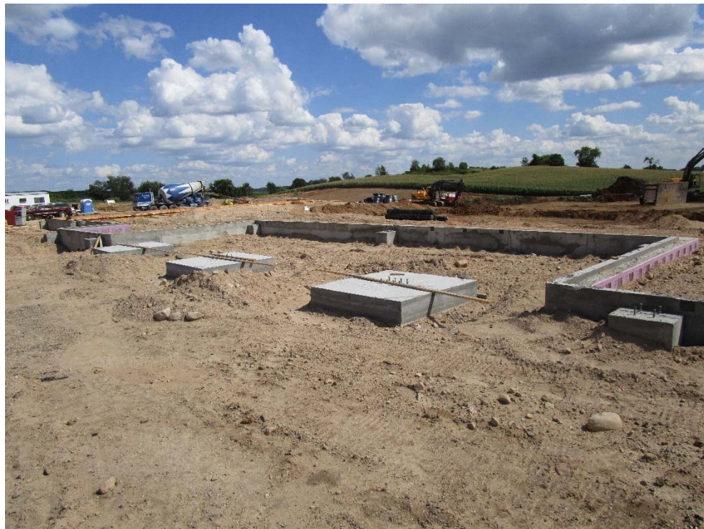
The concrete foundation pictured is the southern outline of the Area B four-classroom pods.
