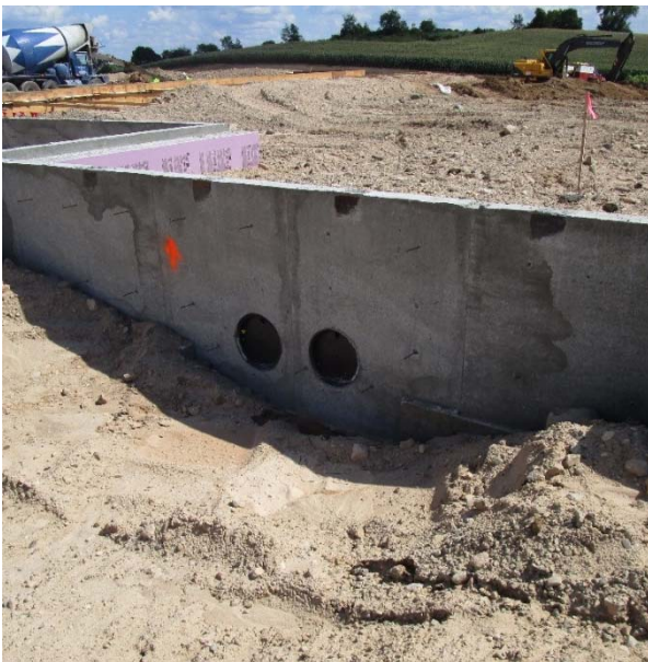
This is where the supply and return lines will enter / exit the building as a part of the geothermal system.
