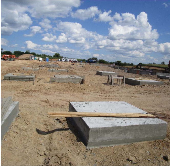
Each square is called a concrete pad, and it is where the vertical steel beams will attach for the structural support of the building.
