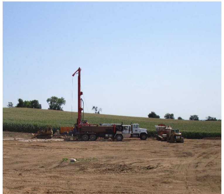
This large drill is now on site to begin the geothermal borefield.
