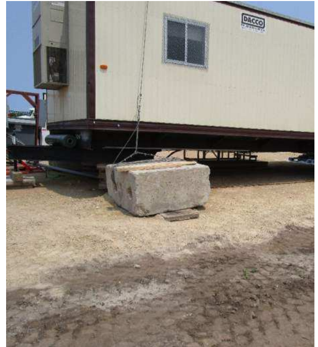
The trailer requires these large weights to prevent tipping from strong winds
