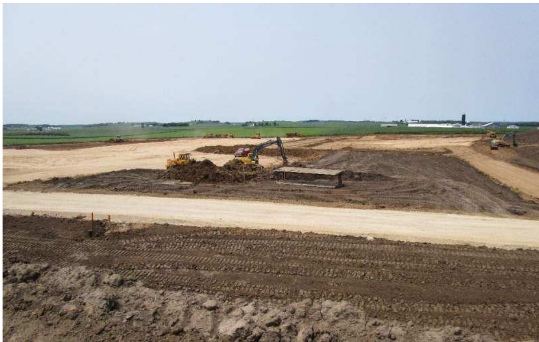
Equipment moving dirt to level the building pad and get ready for foundation work
