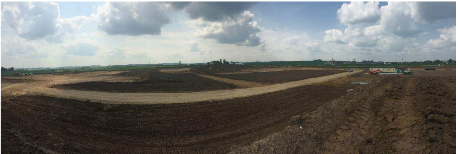
Panoramic image of the entire site including the building location on the left side, with the Findorff trailer on the right side
