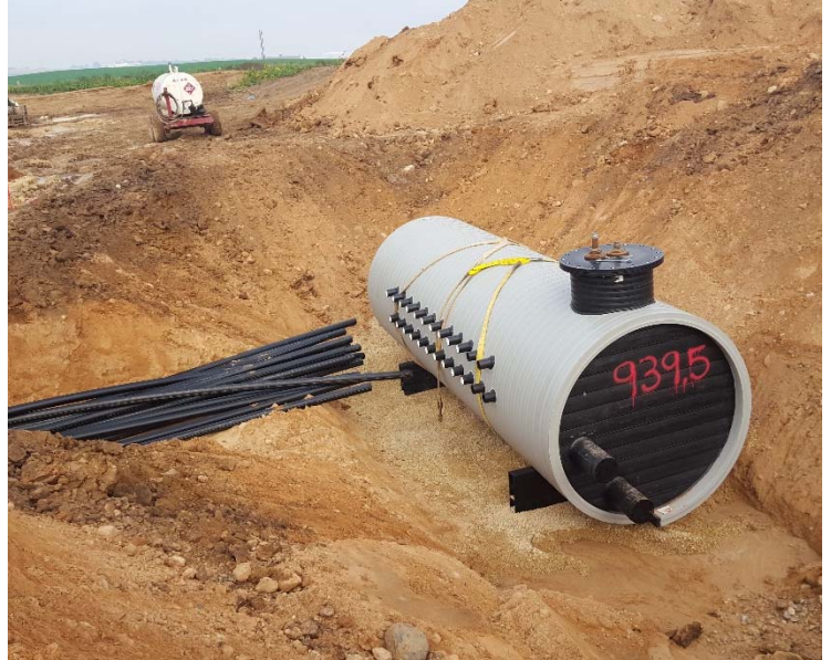
The connection points between the vault and the loop piping covers the left side of the vault, and the supply and returns are on the end.
