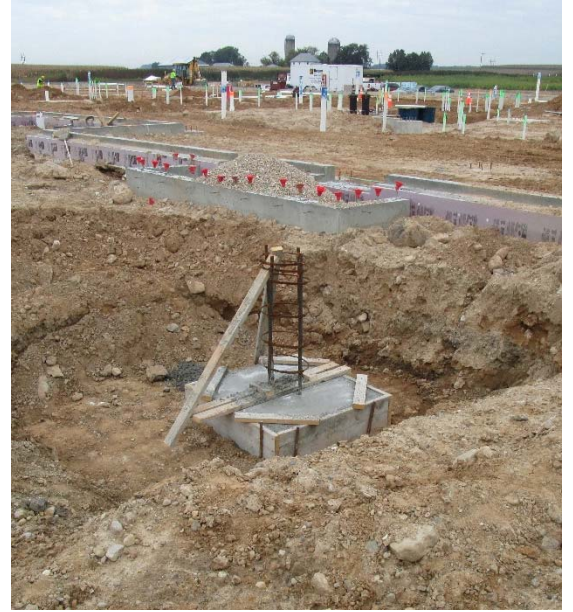
Exterior pads are being poured outside of the perimeter of the building foundation.
