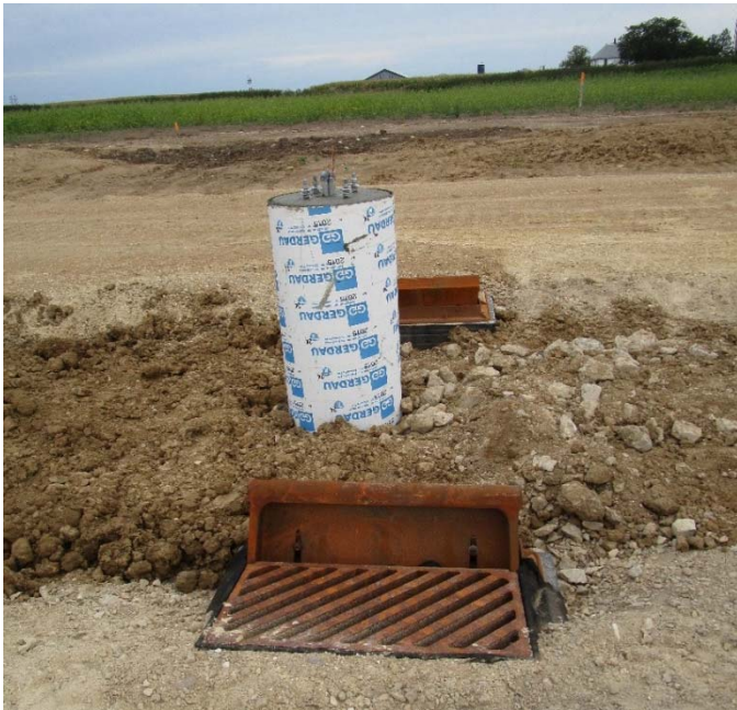
Westphal installed the bases for the light poles this past week. These are located by the main entry road.
