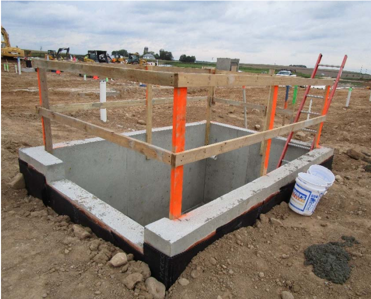
The elevator shaft was poured, and safety railings and gates were attached.
