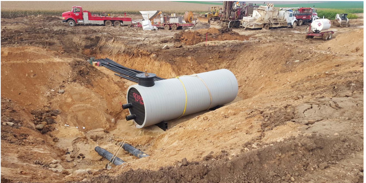
The geothermal vault placed in the ground, and ready for loops to be installed and completed. As you can see, the vault is larger than some of the trucks on site!
