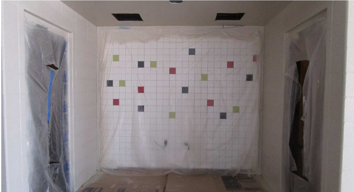
Tile placed as a backsplash for the water fountain area between the boys and girls toilet room.
