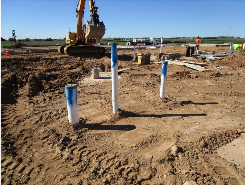
These white pipes with the blue tops are going to be used as storm water drainage.
