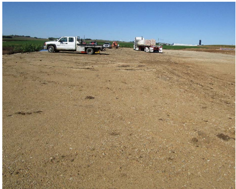
Some of our subcontractors have already been using the new back parking lot.
