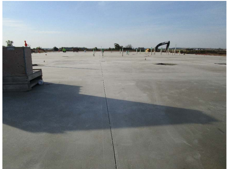
Area A slab on grade is completely done, making it ready for steel next week!
