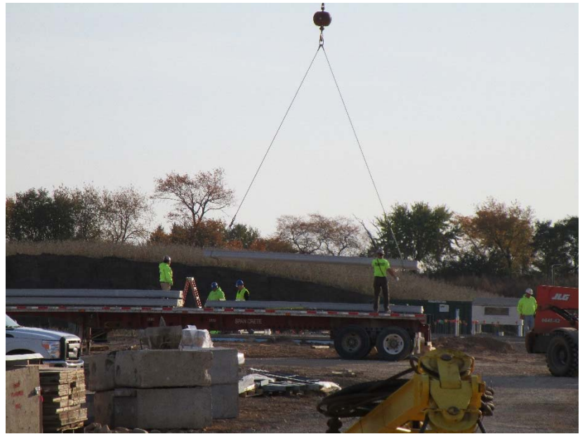
Precast plank is hoisted to be set on the beams of Area B.
