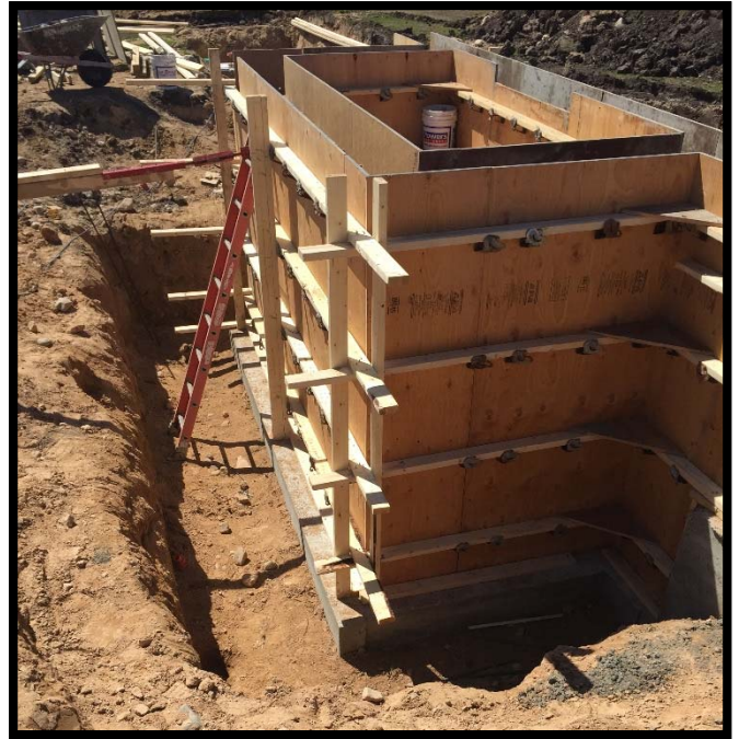
Wall forms constructed by the Findorff crew on the western side of the addition.
