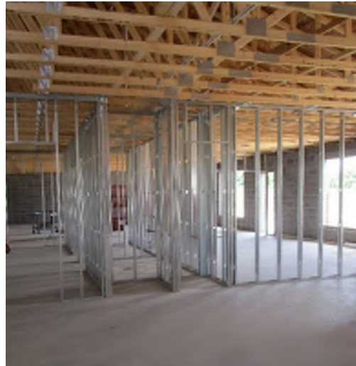
The framing for the kindergarten classrooms was put up this past week.
