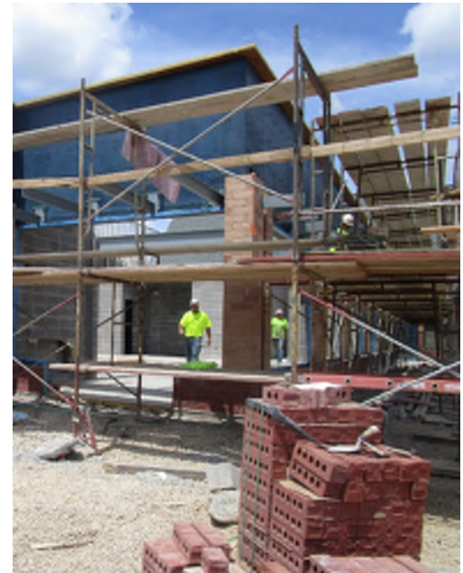
The block at the top of the building are blue because they are weather-proof, ready for the Wisconsin winters!
