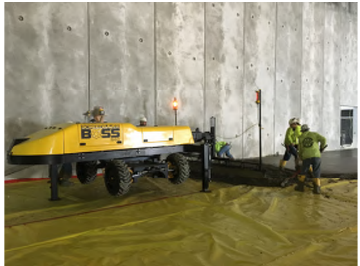
Trying new technology – Findorff concrete crew trying out a new power laser screed to finish the concrete.
