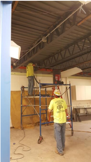
Steel workers are preparing a classroom so that it is strong enough to support a new therapy swing!
