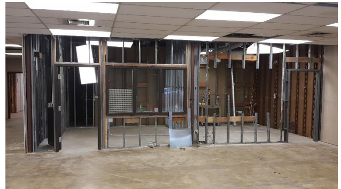
Metal stud framing is coming along nicely. Here is a sneak peek at the new resource rooms on the lower level.
