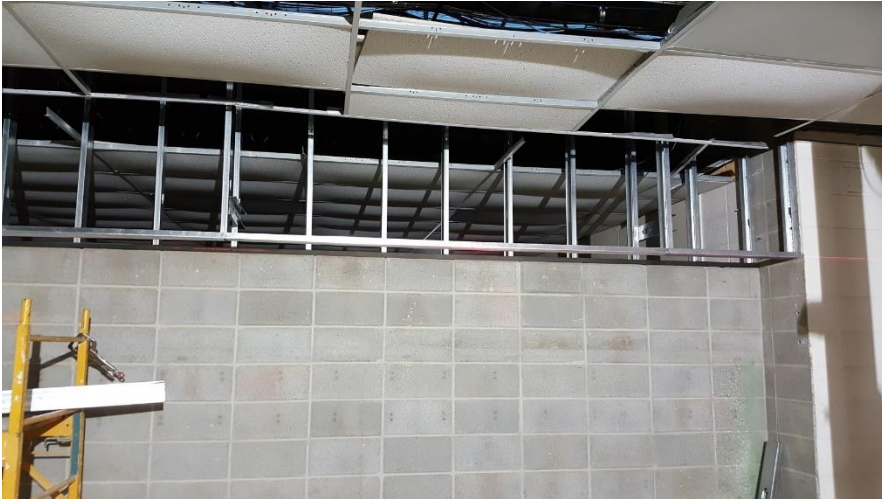
Framing for the open space above the display cases is in progress. It will incorporate the display cases into the hallway really nicely.
