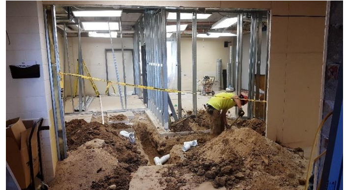
Tradesmen are hard at work getting all the Mechanical, Electrical and Plumbing Rough-ins installed.
