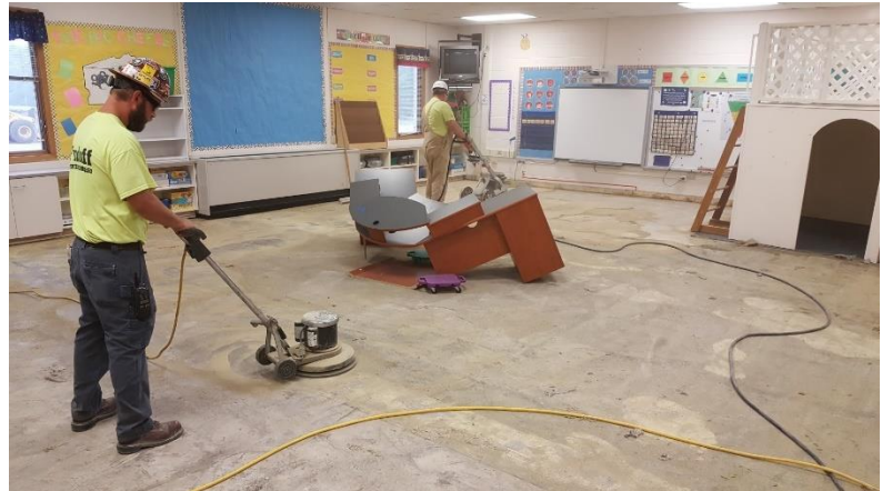
Now that the old carpet is removed, workers are beginning to prepare the concrete for the brand new carpet.
