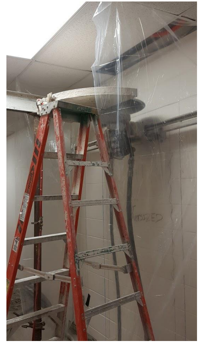
A large saw, similar to that of a Circular Saw, is being used to cut block in order to make the opening for a new doorway.
