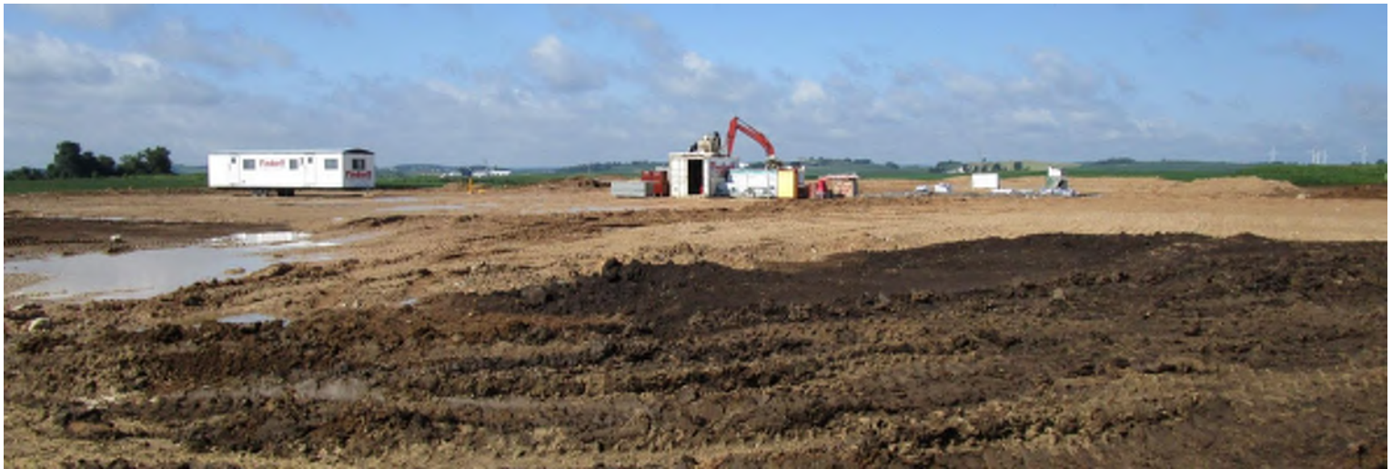
Foundation materials were moved to the new building location. Footings and foundations will begin next week.
