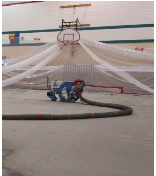
The gym floor was removed, and the area is being prepped for the new floor installation.
