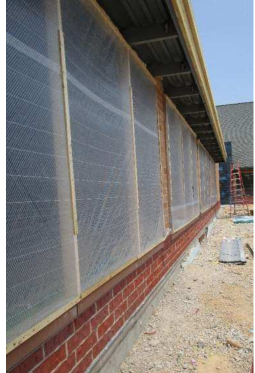
Visqueen is put where the windows will go so drywall can begin next week.
