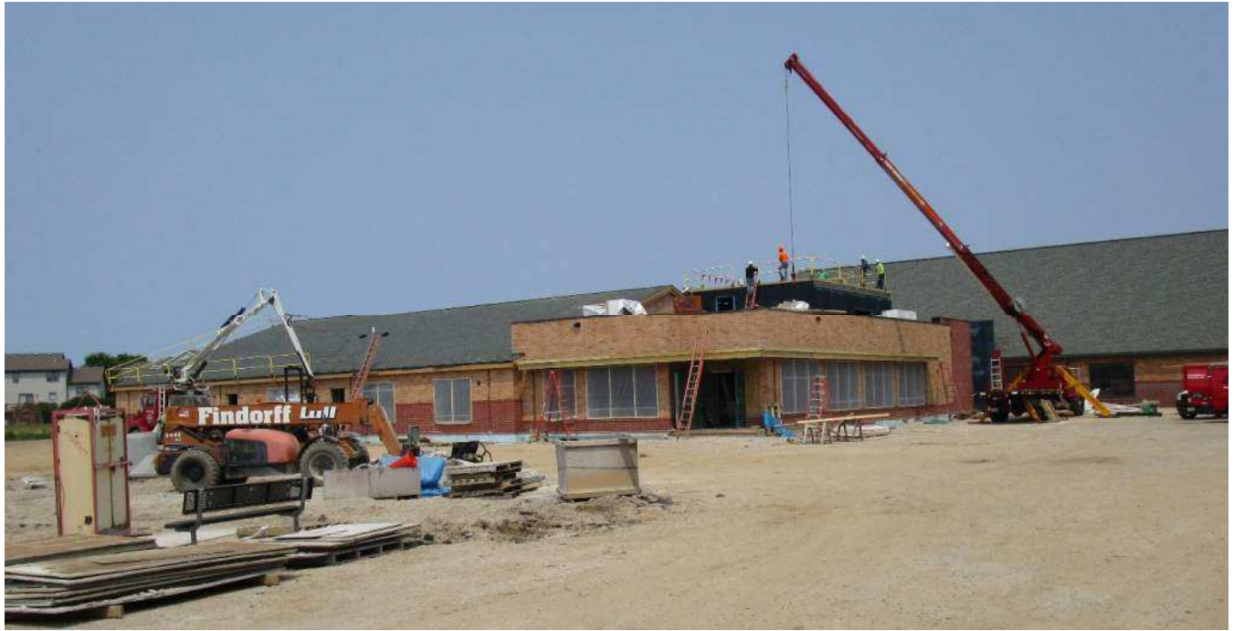
Overall view of the addition with completed shingles, and the early stages of waterproofing completed.
