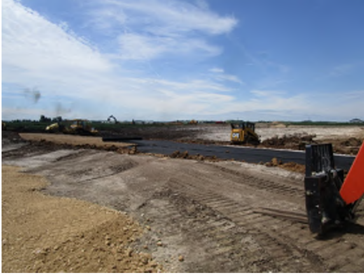
Geotextile fabric being placed before dirt is pushed over it at the new driveway.
