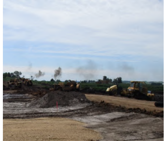
Several earth moving machines working to establish access to the new building location.
