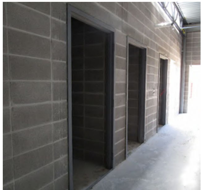
A few door frames have gone in where there will be storage and access to the mechanical mezzanine.
