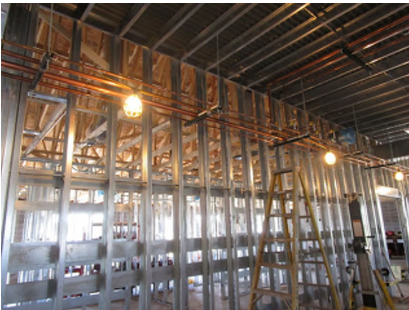
Temp lighting for the construction workers before the permanent lighting is installed.
