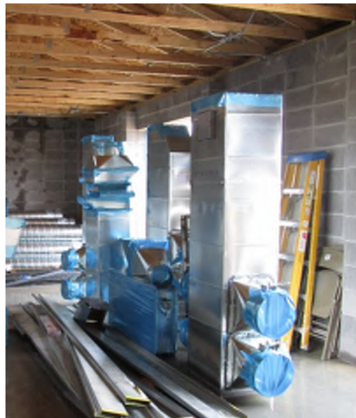
Some of the HVAC ductwork before it was installed.
